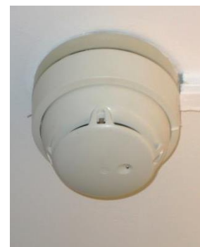
pic. 4.2: smoke detector
