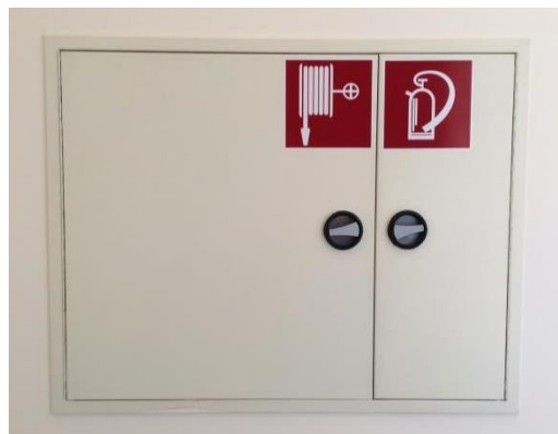
pic. 4.4.1: wall hydrant cabinet (here together with extinguisher)
