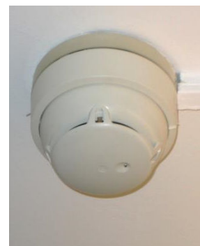
pic. 4.2: smoke detector
