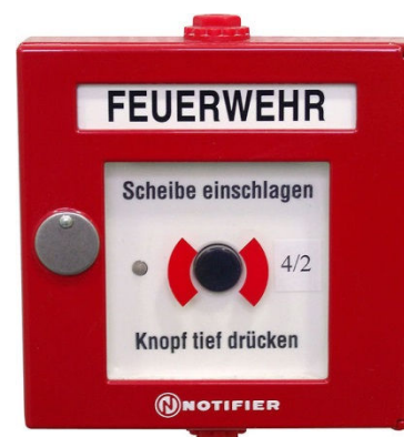
Pic. 4.1: fire alarm button
