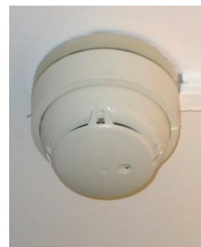
pic. 4.2: smoke detector
