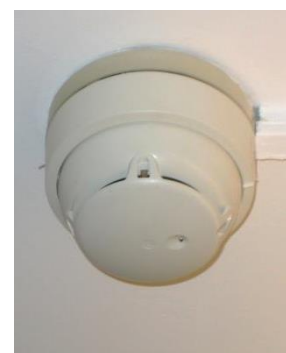
pic. 4.2: smoke detector
