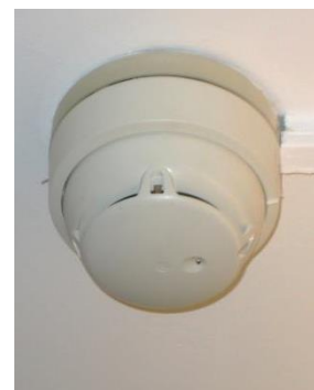
pic. 4.2: smoke detector
