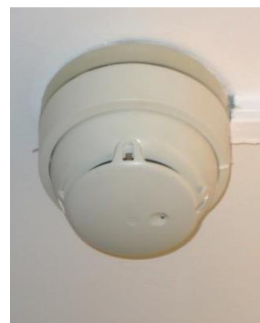
pic. 4.2: smoke detector
