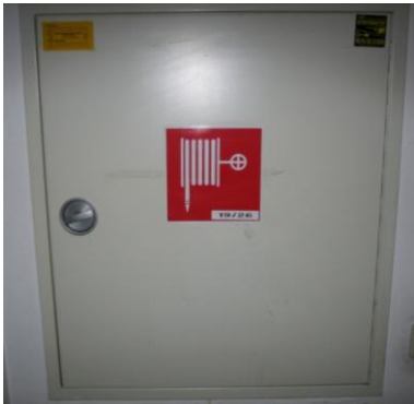
Pict. 5: Fire hose cabinet
