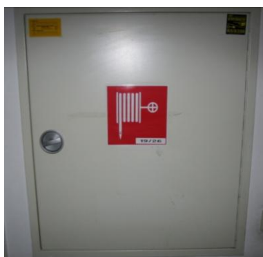
Pict. 4: Fire hose cabinet
