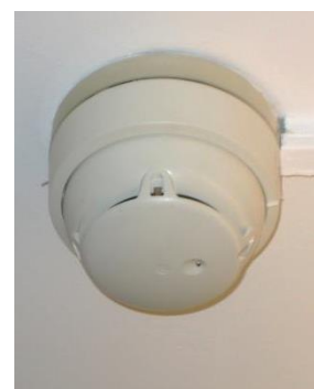
pic. 4.2: smoke detector
