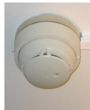
pic. 4.2: smoke detector
