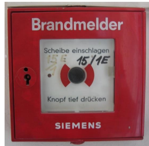
Pict. 1: Fire Alarm Button
