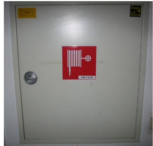
Pict. 4: Fire hose cabinet
