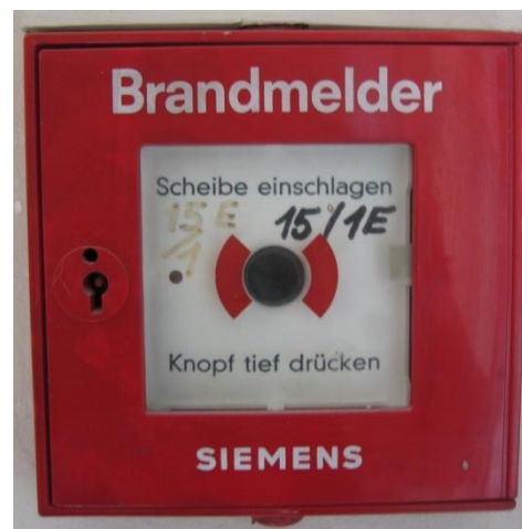
Pict. 1: Fire Alarm Button
