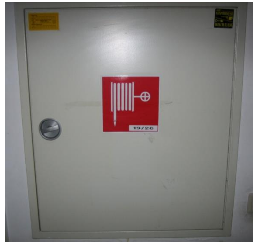
Pict. 4: Fire hose cabinet
