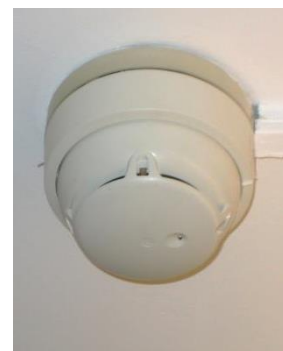
pic. 4.2: smoke detector
