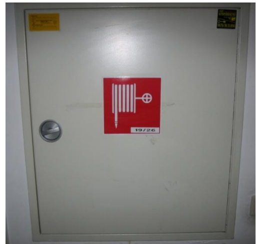
Pict. 4: Fire hose cabinet
