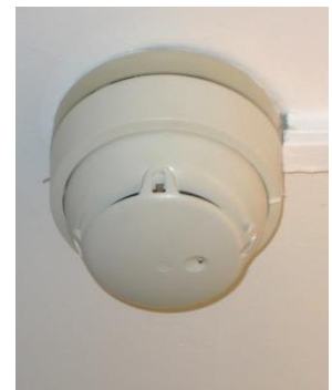
pic. 4.2: smoke detector
