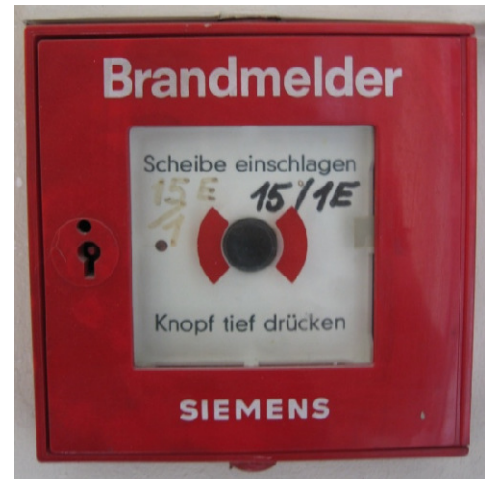
Pict. 1: Fire Alarm Button
