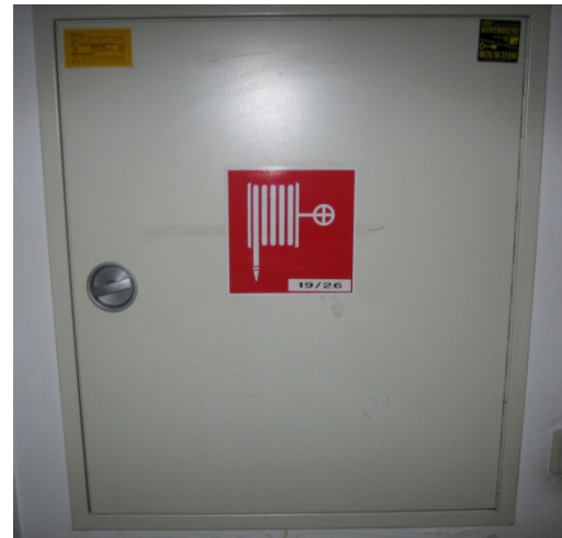
Pict. 4: Fire hose cabinet
