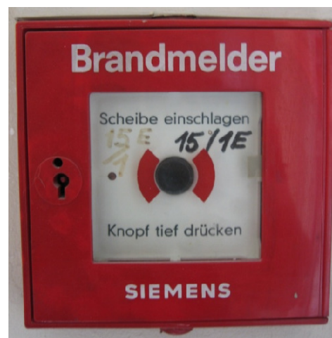
Pict. 1: Fire Alarm Button
